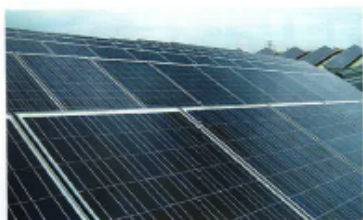
Solar panels on the roof of the Mancaada headquarters
